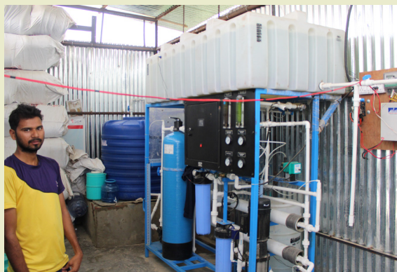
FIGURE 4: RO water-treatment unit in Uttar Pradesh
