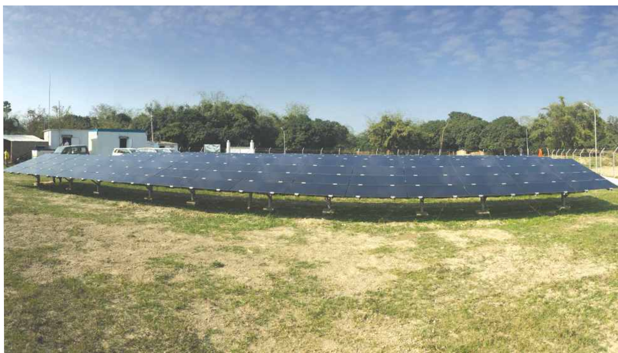
Most Smart Power mini-grids use solar energy, while some use biomass or solar/biomass hybrid technology
